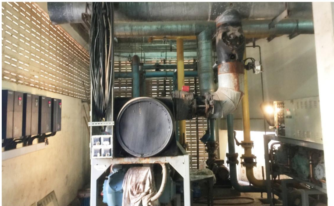
B503D for refrigeration pumps
